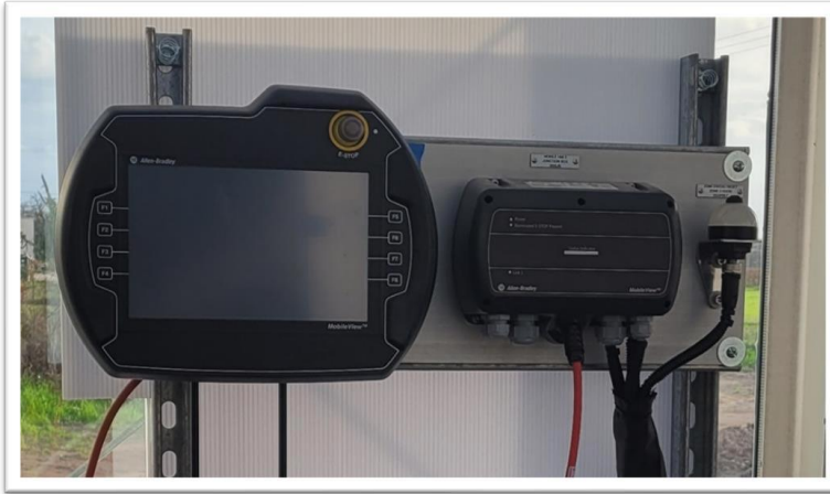
Figure 2: Remote HMI panel and door reset pushbutton
